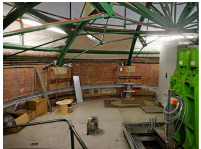
Refurbishment underway in the lift room in the dome of the rotunda at the south end of the Woolwich tunnel. Photo from FOGWOFT
